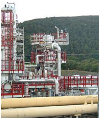
Fig. 1, Test Vessel at Statoil's Karsto Test Facility
