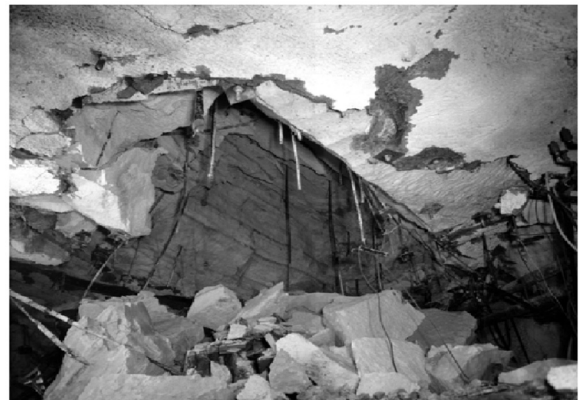
Fig. 1. The blocky nature of the rock mass is evident in the collapse of this cavern in Tuff. This cavern collapsed at stresses below the yield strength of the intact rock mass.
